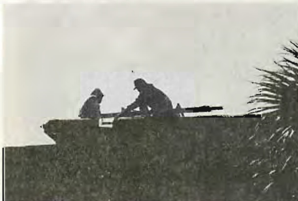
REPAIR--Roofers are silhouetted as they work on the roof of the College Mall.
